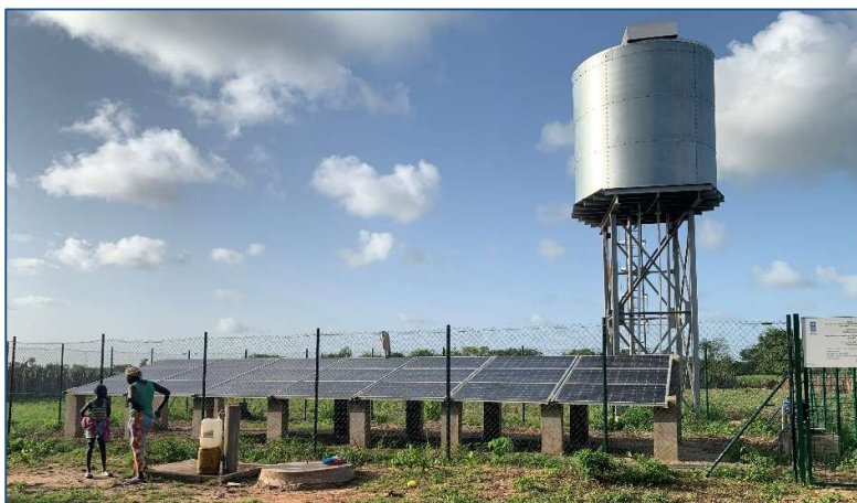
Figure 2. Water supply system provided by PACD
